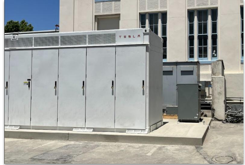
Oakland Tech Battery: Solar Energy Storage
