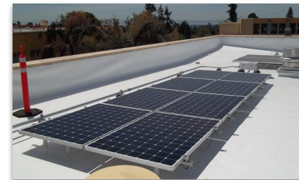
Solar Panel Installations
