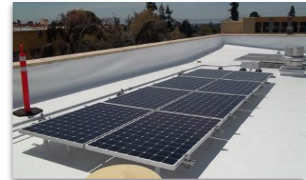
Solar Panel Installations
