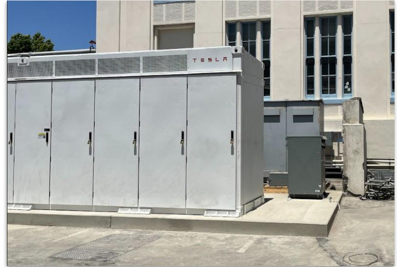
Oakland Tech Battery: Solar Energy Storage
