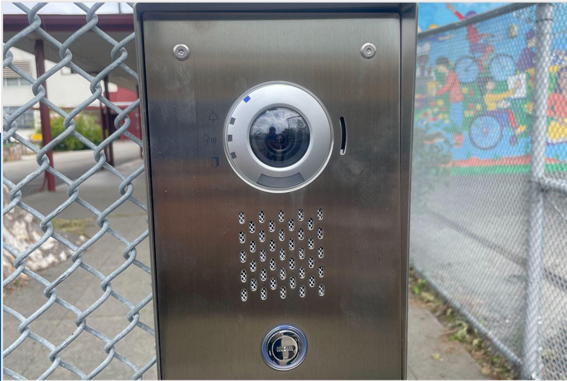
Door entry camera
