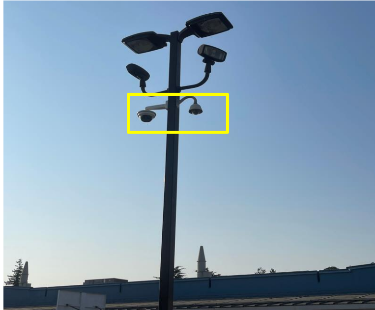
Light pole-mounted security camera
