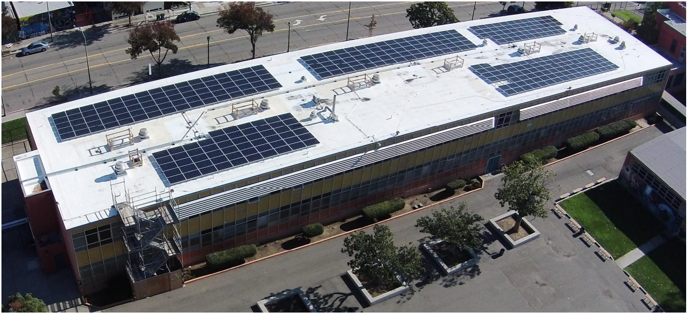
Castlemont High School California Solar Initiative Project
