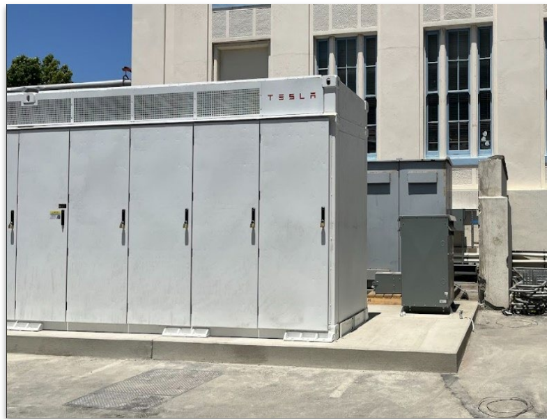
Oakland Tech Battery: Solar Energy Storage
