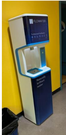
2nd Flowater Unit Installed at Cleveland Elementary
