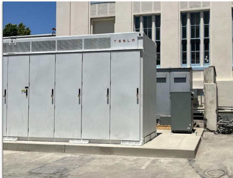
Oakland Tech Battery: Solar Energy Storage
