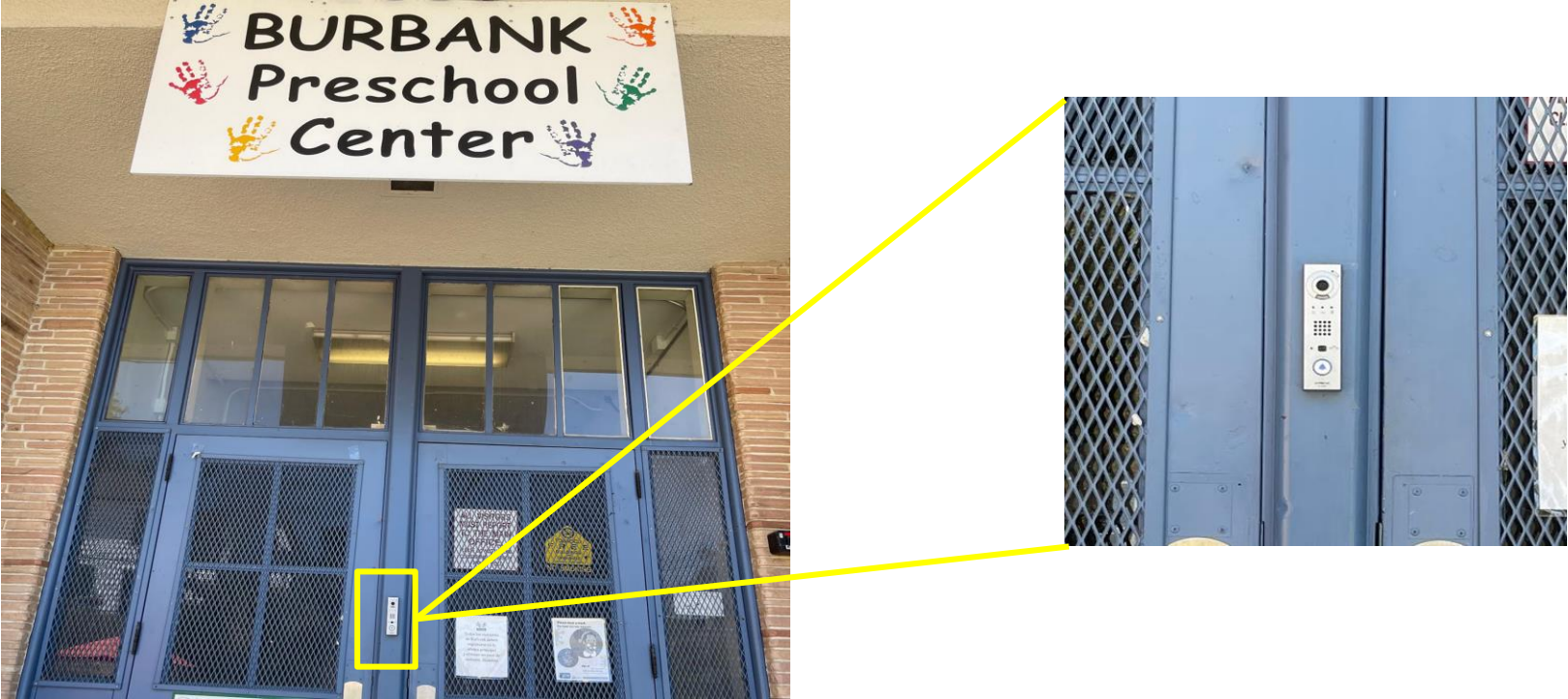
Main entryway area Aiphone IX-DVM door station mounted on center mullion
