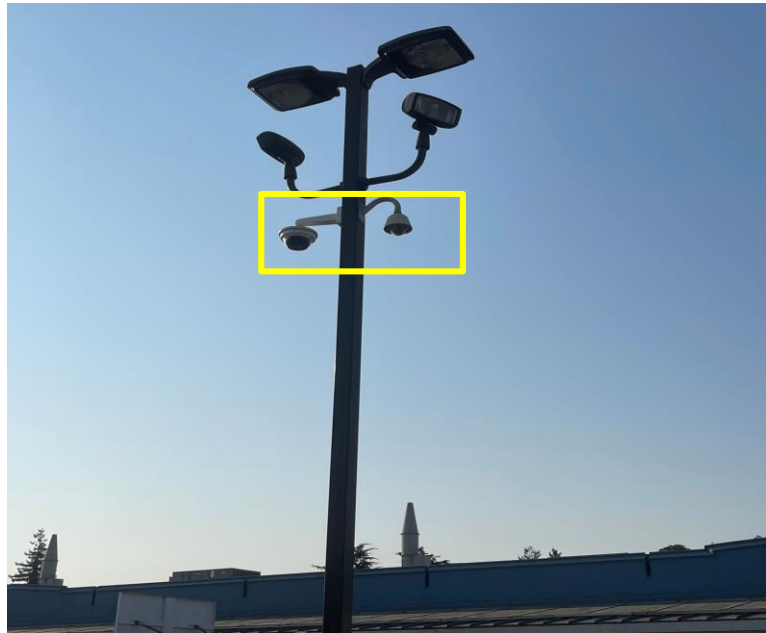
Light pole-mounted security camera
