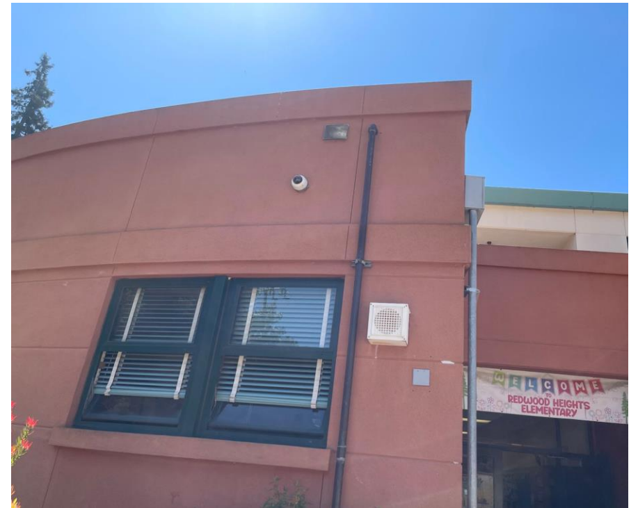
Wall-mounted security camera
