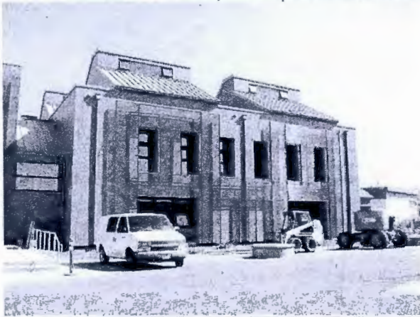
Highland ES New Classroom/MP Building w/ 'Green Screens' and light monitors at rooftop
