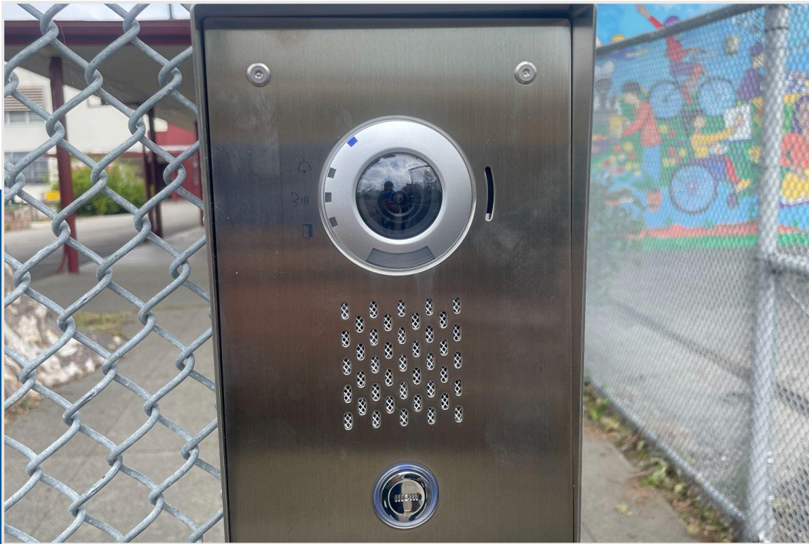
Door entry camera
